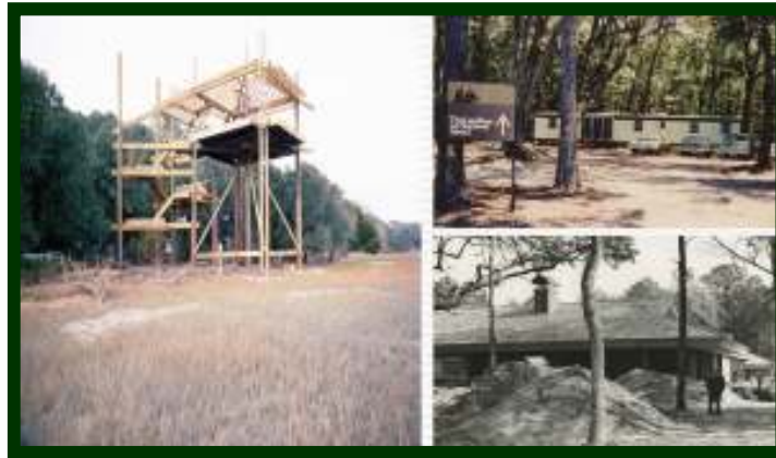
Phase I of The Landings Opened in Sept., 1972. Tower & Marshwood Clubhouse Under Construction; Temporary Sales Office in Modular Unit
